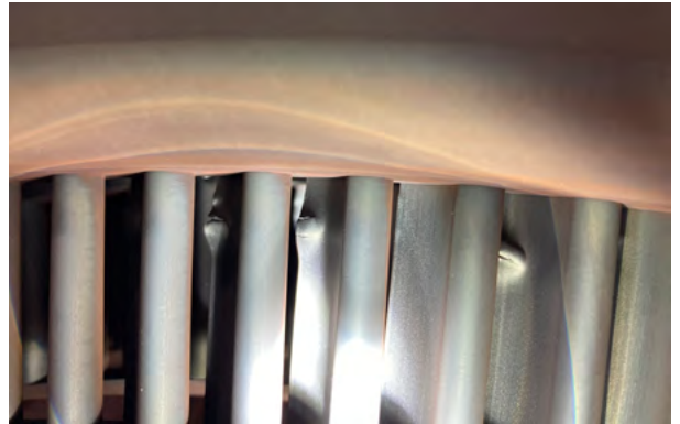
▼ Blade damage caused by foreign particles
