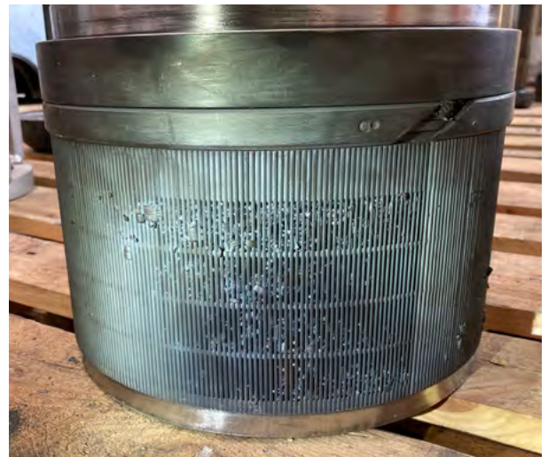
▲ Steam strainers full of foreign particles with some already going through into the turbine
